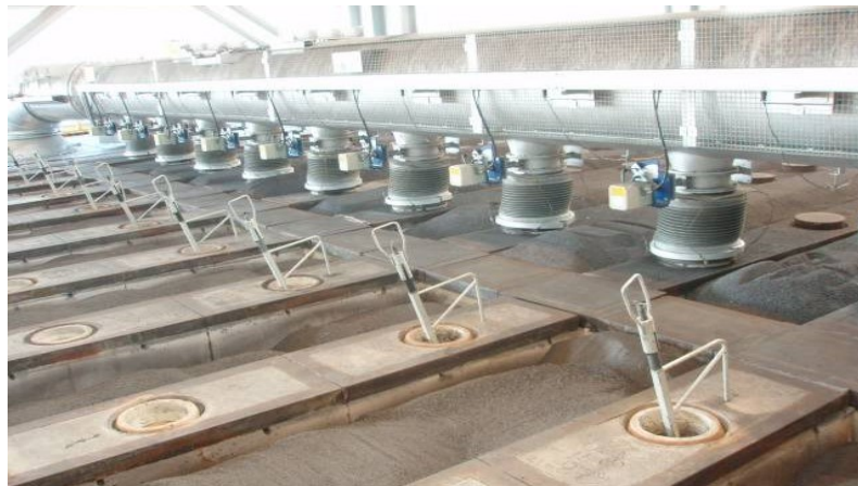
Figure 6. Front of the exhaust ramp: dead section (properly filled with required quantity of packing coke).
